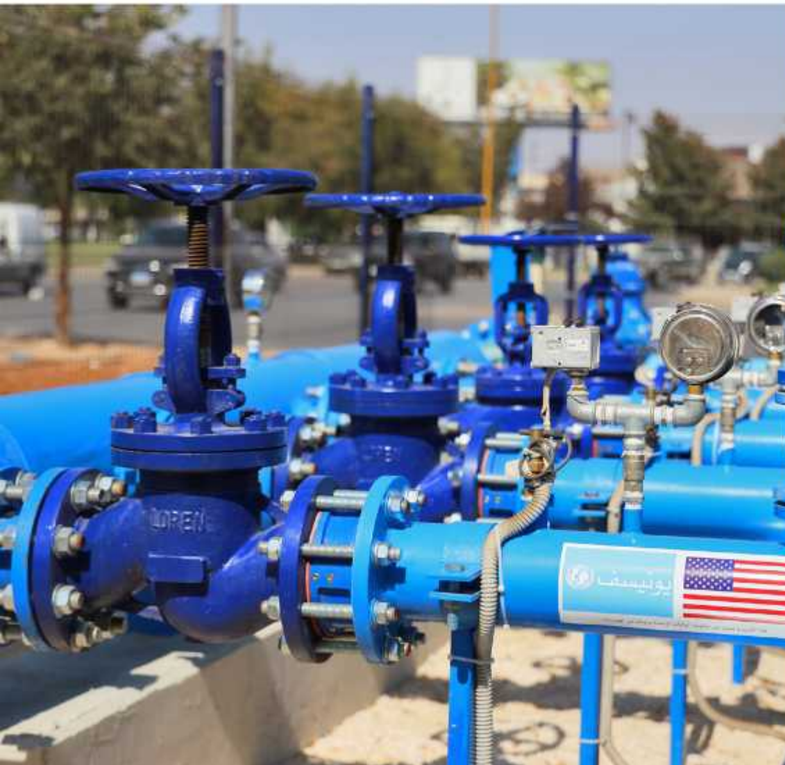
The construction of the Zahle pump station in Lebanon was carried out in cooperation with the Bekaa Water Establishment. It improves access to water for both Syrian refugees and the communities hosting them.
