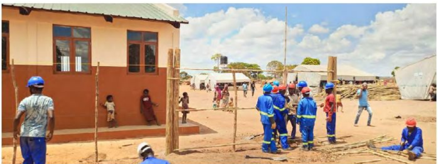
The building of the Maroccane school fence in the CFW programme in Mozambique. © IOM 2022
