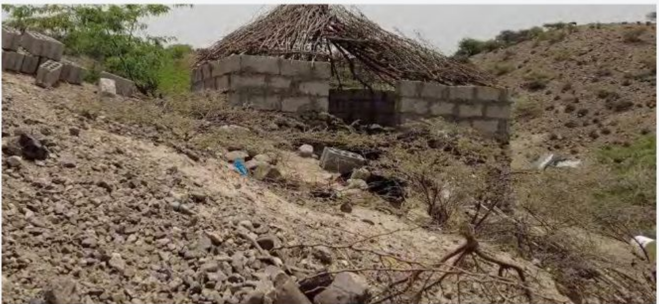
Hussein's partially constructed shelter he is building for his family in Ta'iz with materials purchased from cash support provided by IOM and the Yemen Humanitarian Fund. © IOM 2022/Mohammed MAJED
